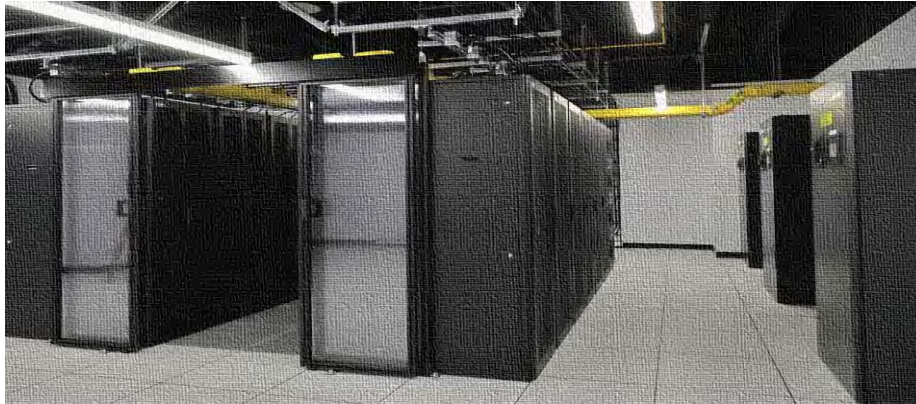
Patriot.Online private datacenter and secure infrastructure
